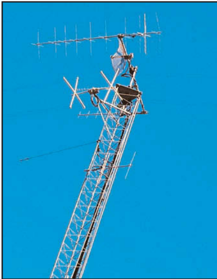
Figure 2—Looking up the tower at the center spreaders of the Cage antenna at W1AW.
